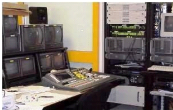
(The system of Coming Soon Television)
