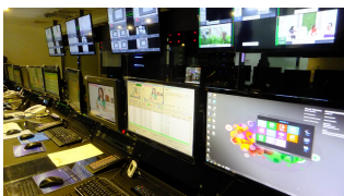
U-Life master control room
