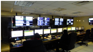
U-Life master control room
