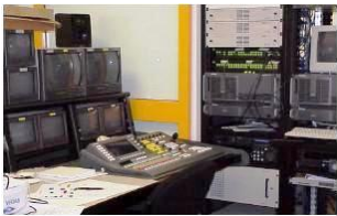
The system of Coming Soon Television
